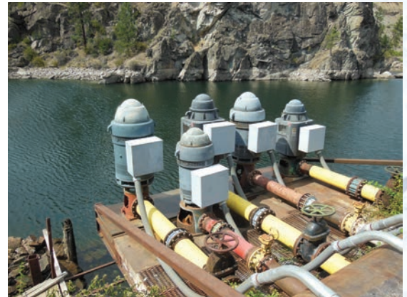
Quadplex River Booster System.
